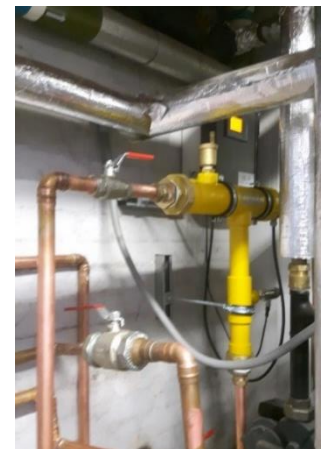
Protex installation in actual buildings
