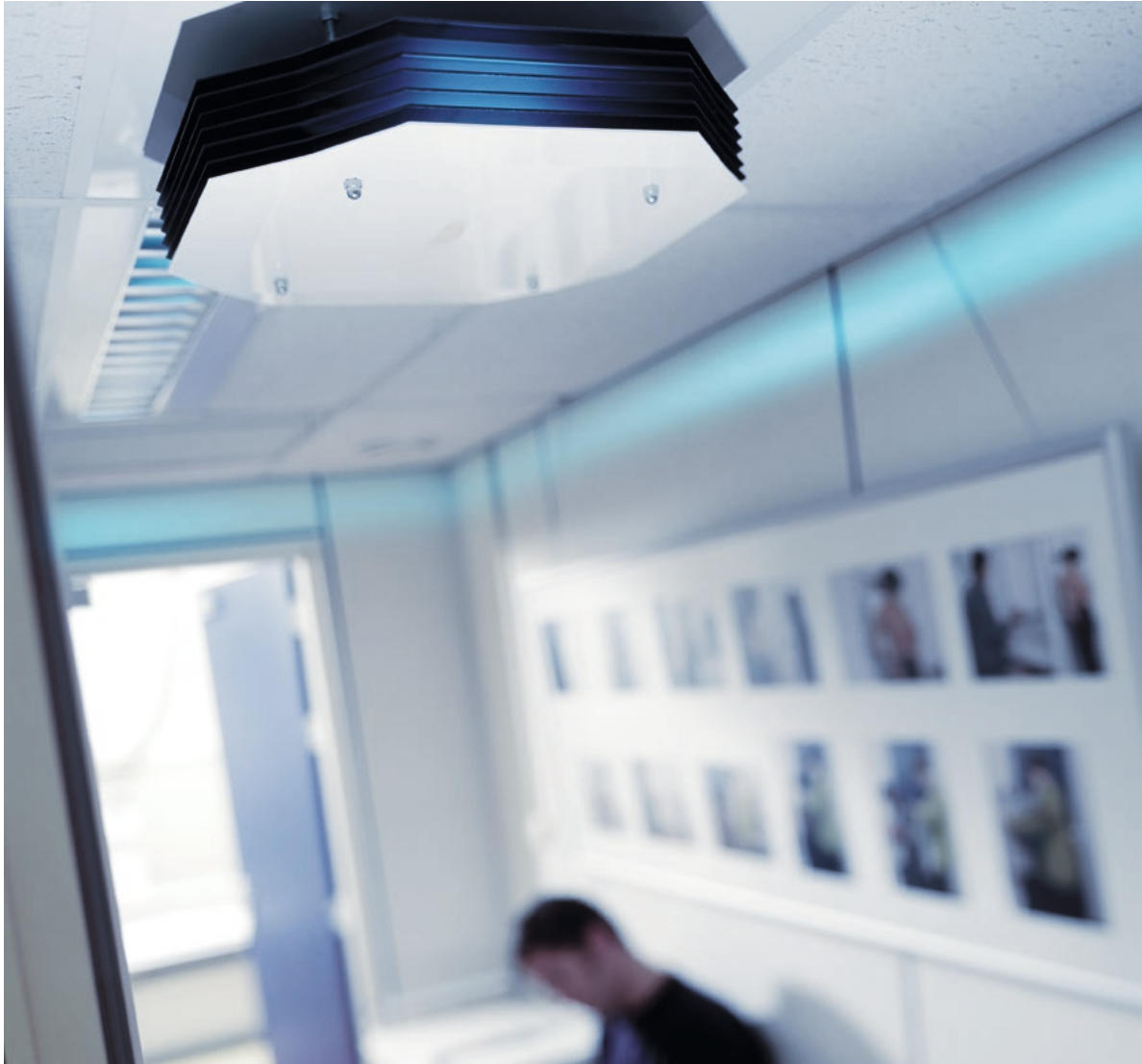
Hospital waiting room with UVGI installation courtesy of Signify
