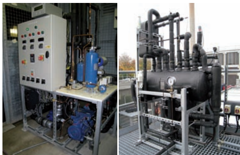
Subcritical CO 2 refrigeration
