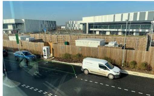
Figure 26: Gridserve Forecourt inverters providing power to DCFCs from grid source and battery storage.
