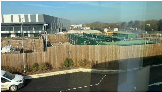
Figure 25: Gridserve Forecourt 6mWh battery in shipping containers, storing input from a 5mW 33kV grid connection.
