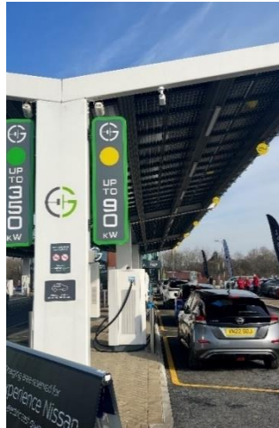
Figure 6: Rapid + Ultra-Rapid Charging Spaces at a Gridserve Forecourt, with overhead Solar PV.
