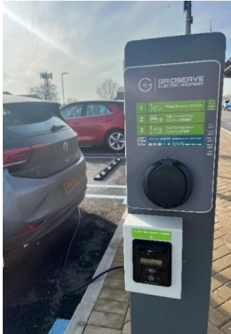
Figure 5: AC (Level 2) Fast Charging at a Gridserve Forecourt. A contactless bank/credit card can be used to charge.
