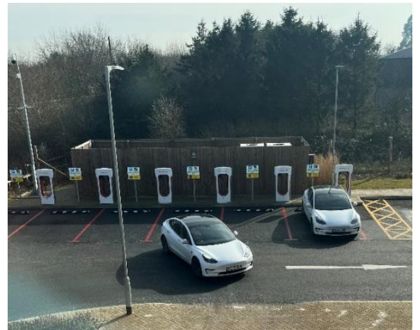
Figure 7: Tesla Superchargers at a Gridserve Forecourt.
