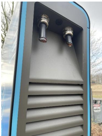
Figure 1: A vandalized DCFC
