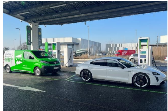
Figure 12: A Vauxhall Vivaro-e operated by OVO Energy, and a private Porsche Taycan charging at 350kW (capable) DCFCs at a Gridserve Forecourt
