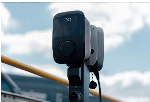
Figure 17: 22kW EO Genius 2 AC EVSEs at an Amazon charging depot. Source: EO Charging
